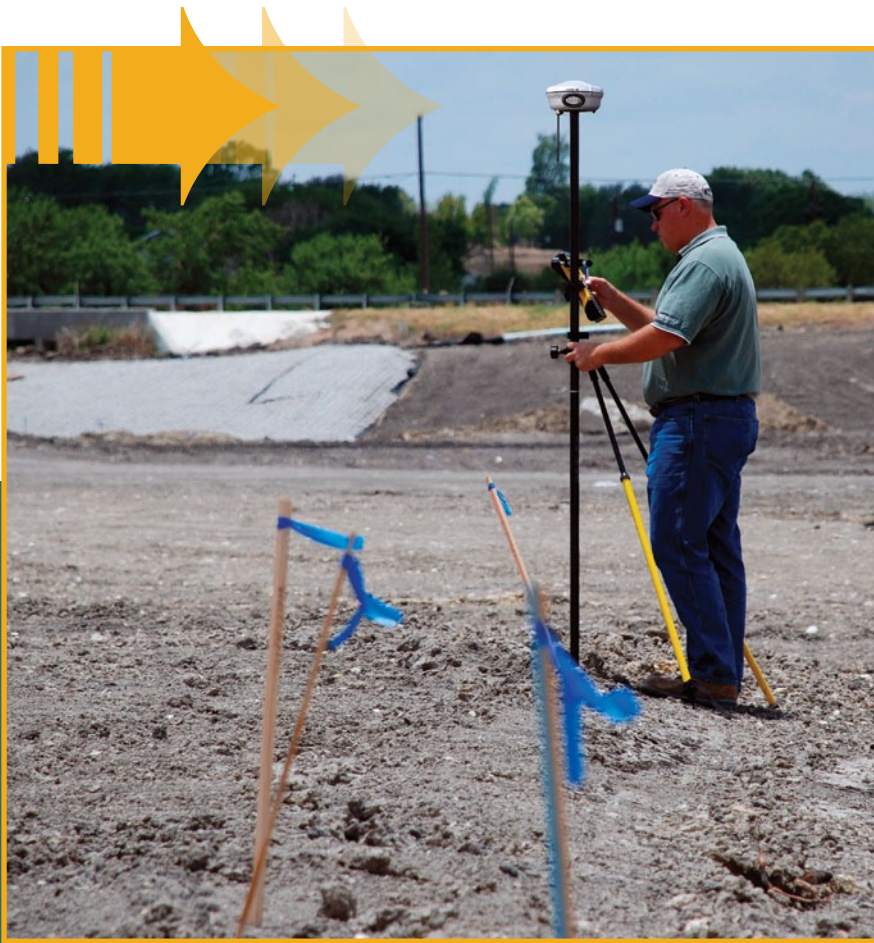
A surveyor puts the Trimble system to work on a project site. The proliferation of cellular and WiFi service provides increased capability for field-to-office collaboration using Trimble Assistant.
